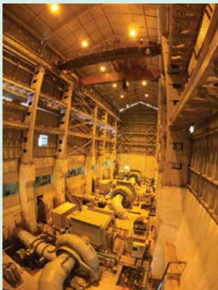
DIKSHI 24 MW SHP-Power House
