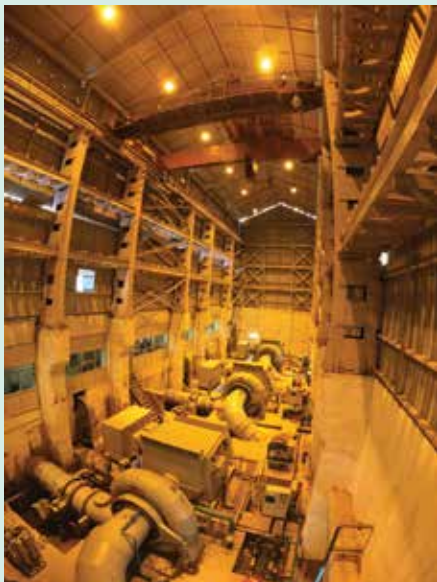
DIKSHI 24 MW SHP-Power House
